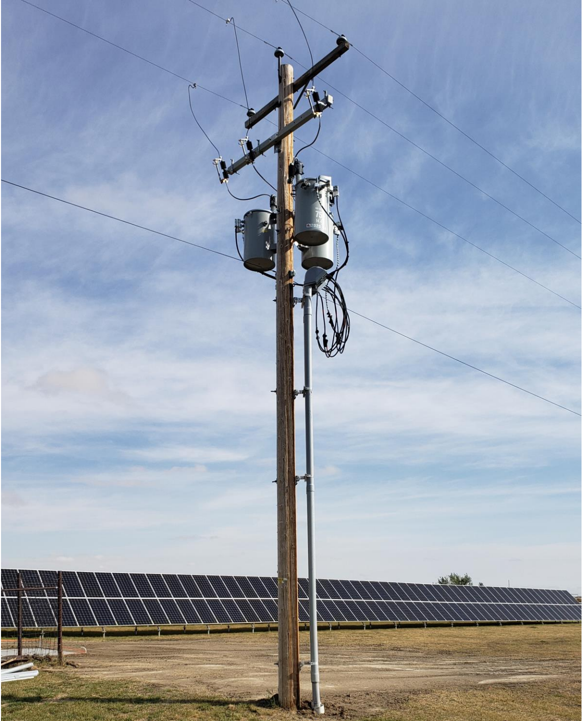
New Fortis transformer
