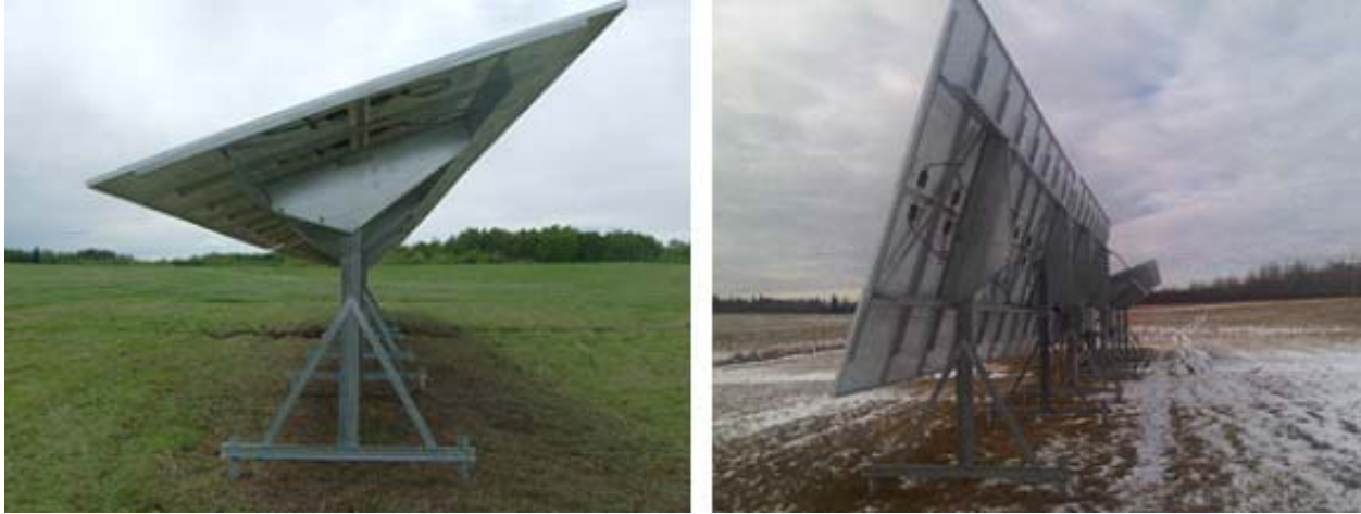
Figure 4 - PV Array (summer and winter positions)
